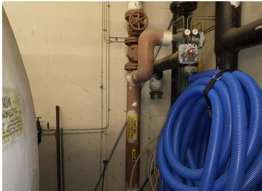
Pipe Insulation – Warning Labels Affixed
