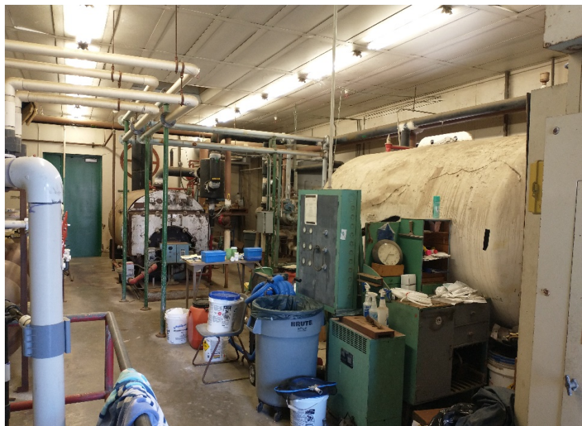
General Pool Equipment Room
