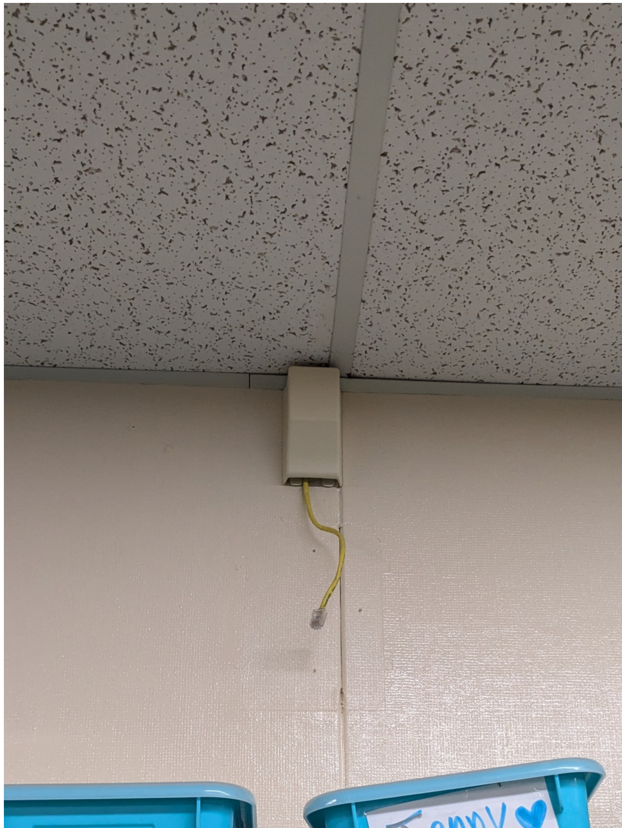
PIC. DETAIL - ABANDONED AP MOUNT AND CABLE (TYP.)
