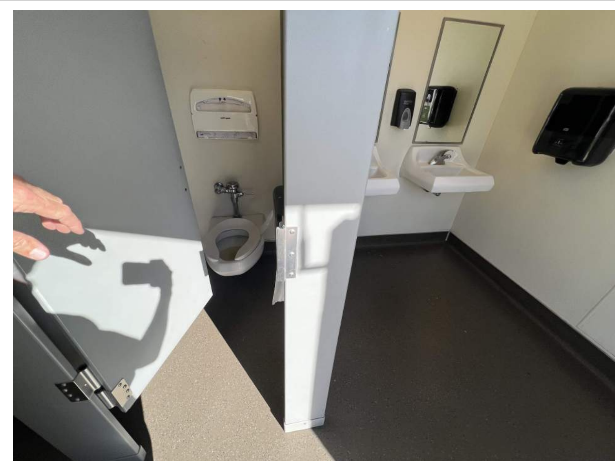
P-102 GIRLS RESTROOM -E. FIELD VERIFIED CONDITIONS
