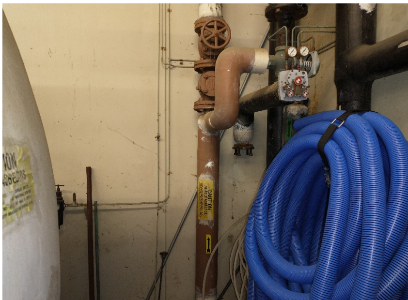
Pipe Insulation – Warning Labels Affixed
