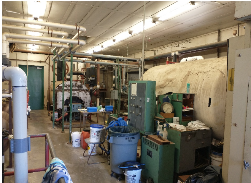
General Pool Equipment Room
