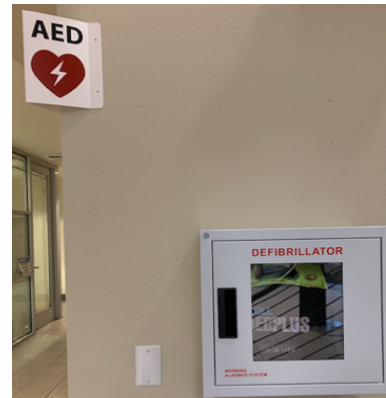
One of 138 AEDs across 81 SCUSD campuses maintained by Health Services
